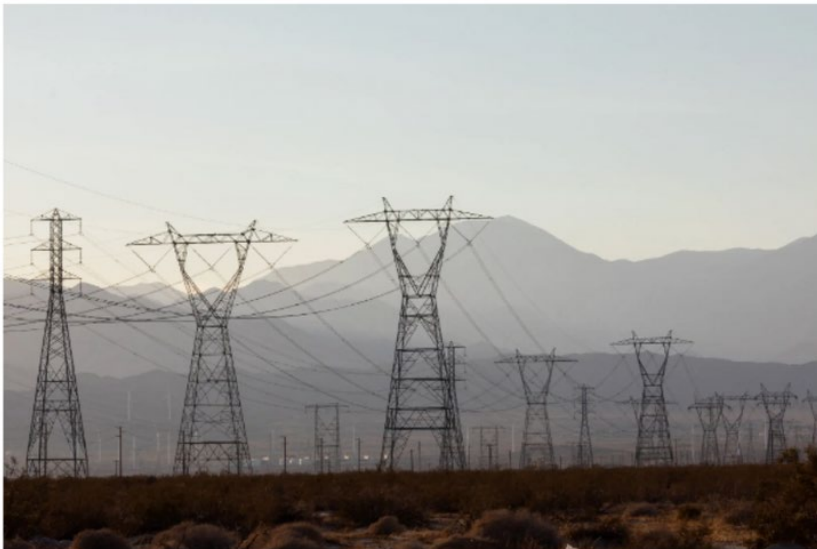
Power lines in Cathedral City, Calif., during the heat wave on Tuesday. Alex Welsh for The New York Times
