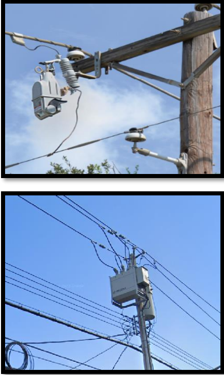
Automation to detect and isolate faults, reducing outages
